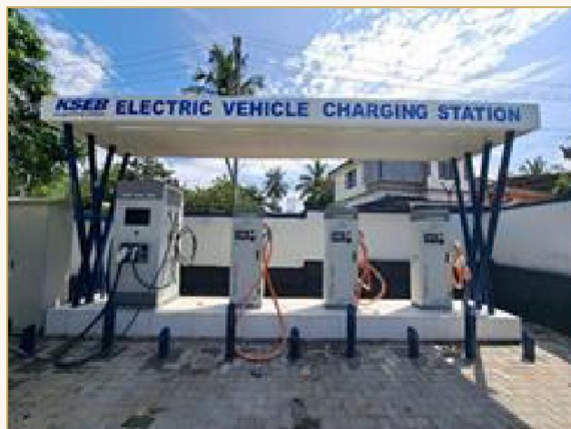
EV CHARGING INFRASTRUCTURE IS EXPANDING ACROSS THE STATE
